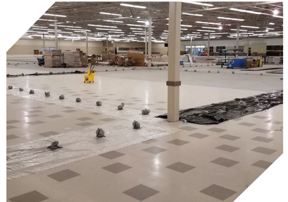
Hydrophobic expansive polyurethane grouting to fill voids under the slab at an industrial facility.
